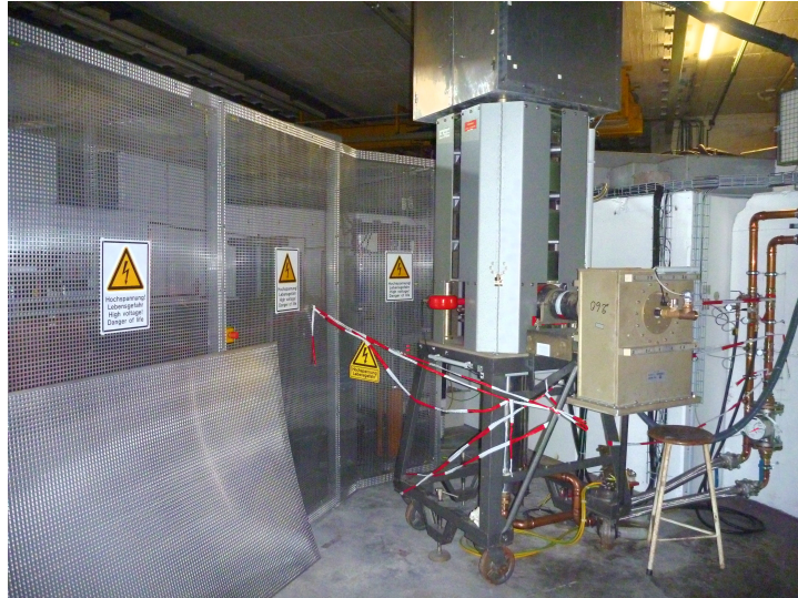
Figure 3.13 – Klystron site with high voltage power supply on the left site and klystron on the right. The rectangular incoupling in the WR1800 waveguide can be seen on the right side of the klystron.
